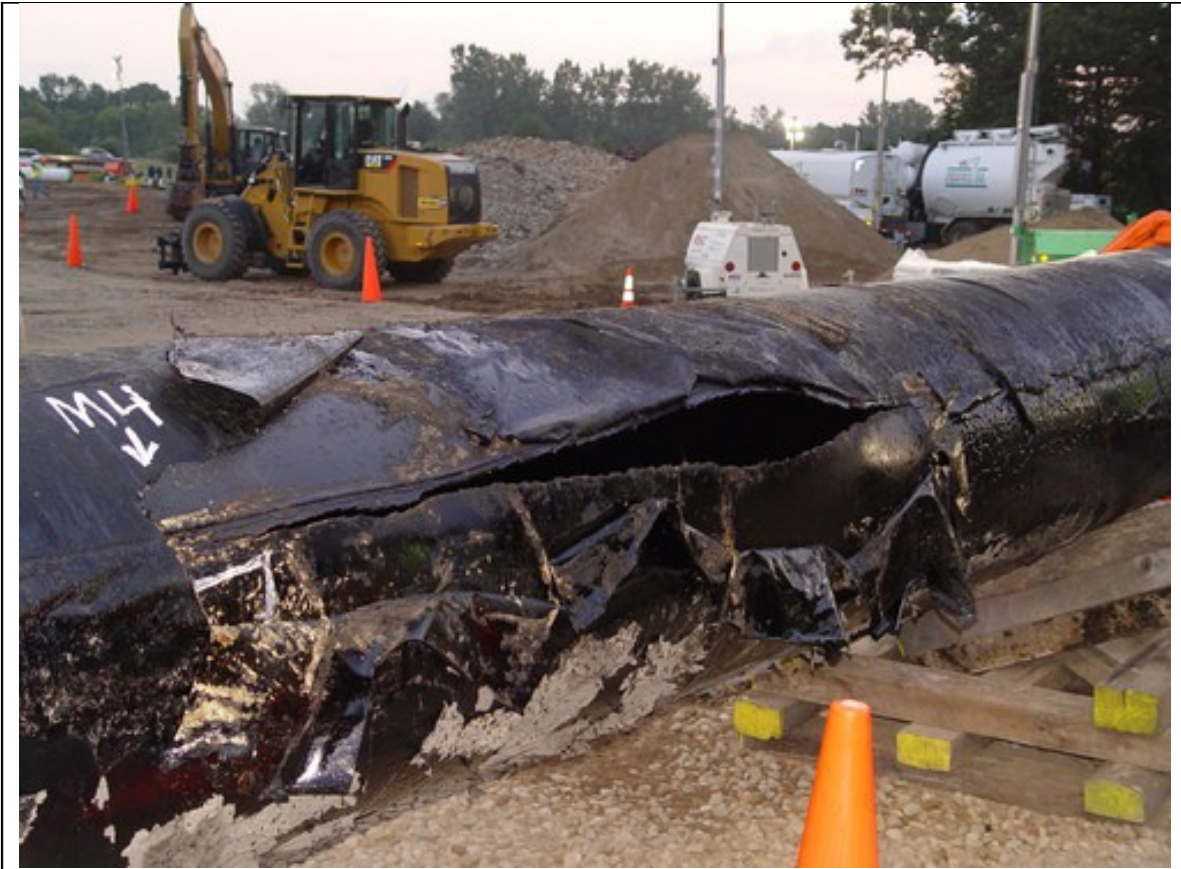
Enbridge's Oil Pipeline Breach Near Kalamazoo, MI
